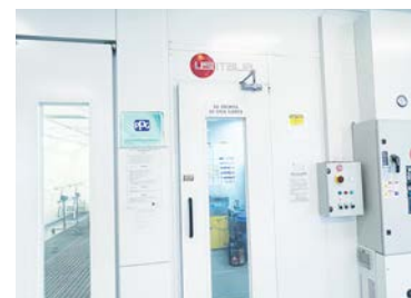
Moppert Brothers purchased two booths and a paint mixing room from USI Italia for its Northfield location.
