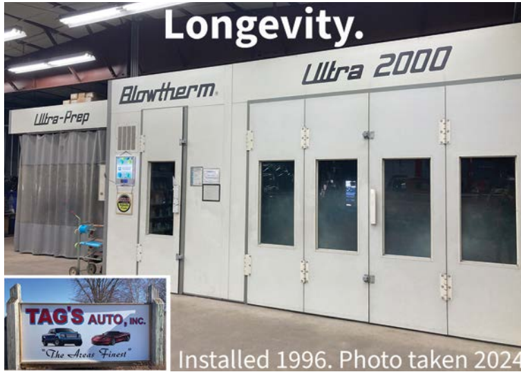
Proper maintenance has kept this 1,700,000-hour Blowtherm spray booth and prep station combination running like the day it was installed at Tag's Auto Inc. in Clintonville, WI.
